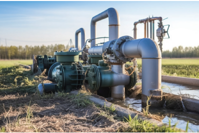
Constant pressure water supply
